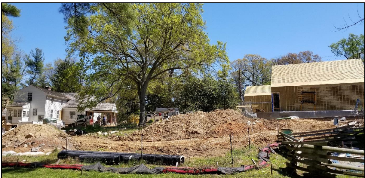
Josiah Henson Visitor Center and Museum under construction next to the Riley Plantation house.
