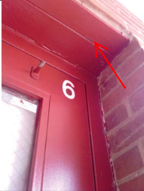
Picture 17: Red Metal Door Lintel
